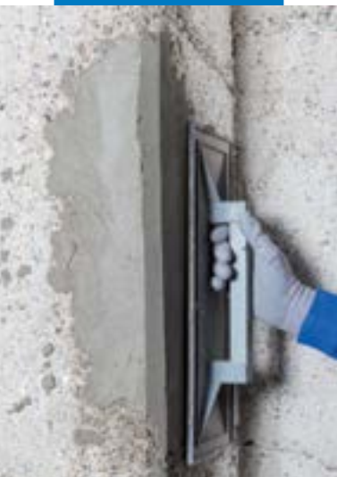
Floating the surface of Planitop Smooth & Repair R4 ZA to create a smooth finish
